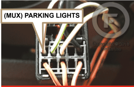
③ At parking light switch.
