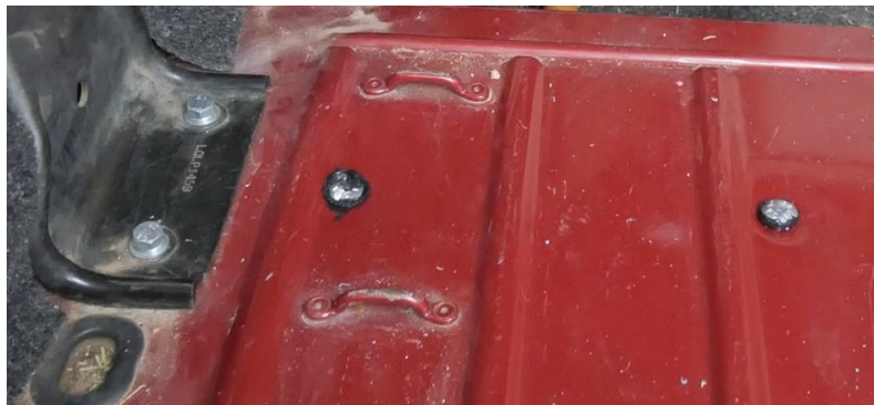
Figure 14 – Ribbed Neck Bolt installation (Cross Section of Floor & 1999 TJ Shown w/ Bolts Installed)
