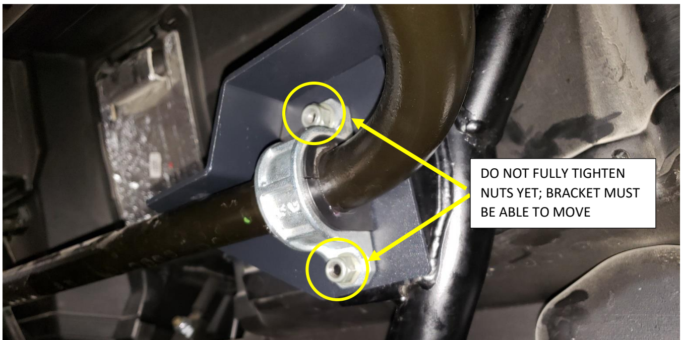
Figure 14 - Driver Side Sway Bar Nuts/Bolts with Air Tank Bracket Inserted
