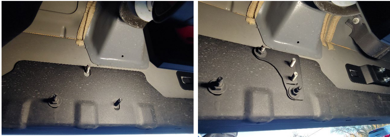
Figure 35- Driver Horn Bracket, Installed
