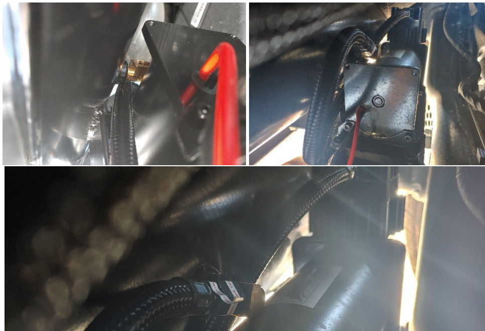
Figure 14- Tank / Compressor Plumbing
